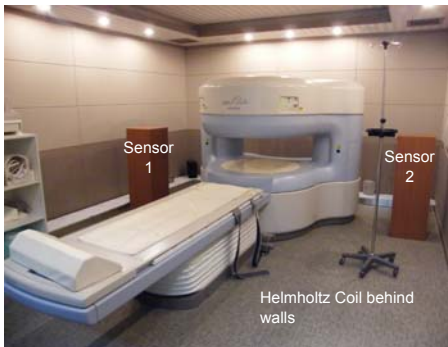
Hitachi MRI Elite 0.3T Yunse Hospital, South Korea Interference from cars and subway trains Without MagEclipse: 15 mG (0.1 - 2 Hz) With MagEclipse: 1 mG (0.1 - 2 Hz)
